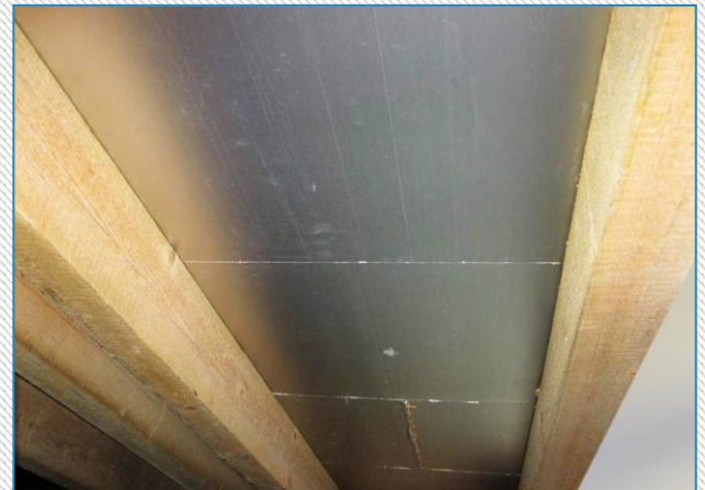
Picture 1: Inside of the pitched roof with the rafters and the insulation layer
