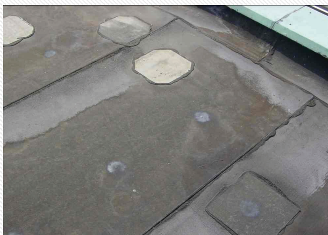
Figure 1: Example of a damaged roof
