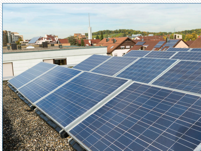
Figure 3: Solar panels on a flat roof (source: IVPU)
