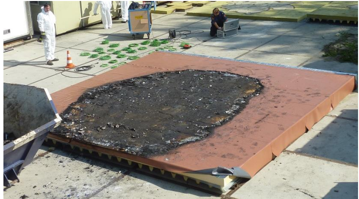
Photo 33 Overview of the burnt roof waterproofing sheet.
