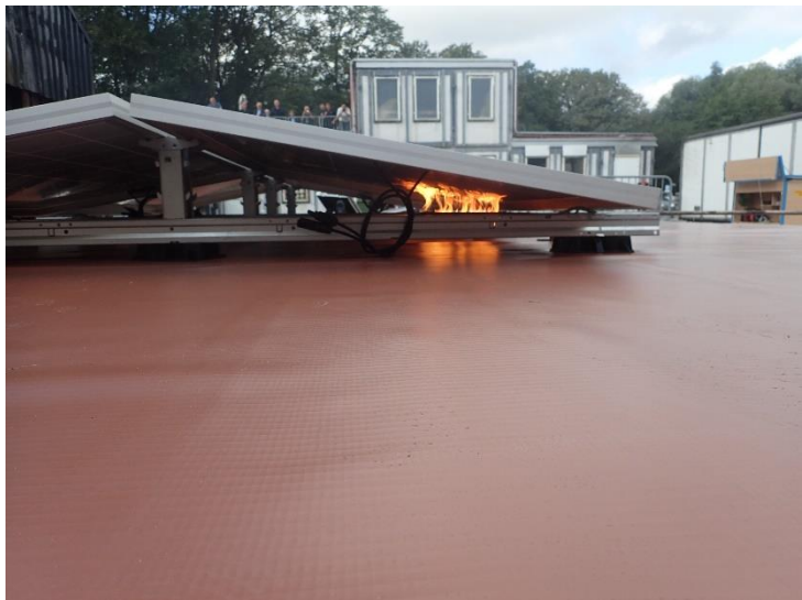
Photo 6 The gas burner has been ignited (time 10:11).
