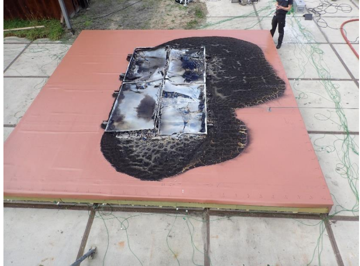
Photo 13 Overview of the burnt roof waterproofing sheet including PV modules.
