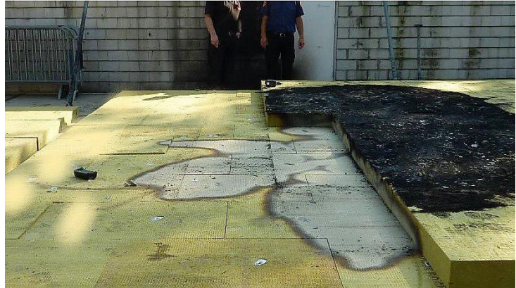
Photo 16 Overview of the burnt section of the MW insulation (top layer and underlayer).
