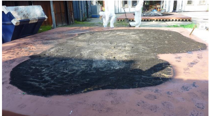
Photo 14 Overview of the burnt roof waterproofing sheet.
