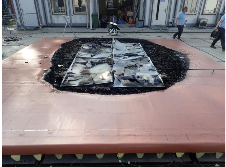
Photo 32 Overview of the burnt roof waterproofing sheet including PV modules.
