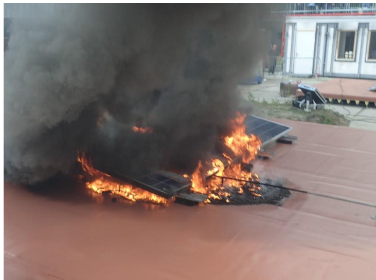
Photo 9 The fire is spreading backwards outside the PV modules (time 10:14).
