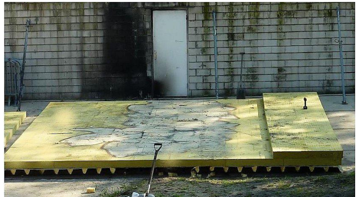
Photo 18 Overview of the burnt section of the MW insulation (underlayer).
