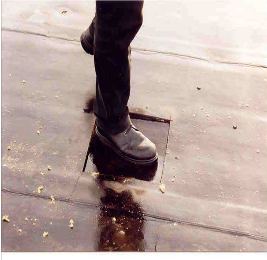
Figure 2. The MWR insulation has become soft, due to (excessive) pedestrian traffic. Various leaks (caused by penetration by screw heads) have been repaired, but new perforations are already starting to appear.
