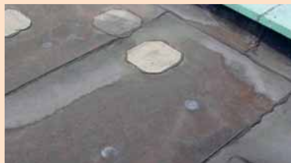
Example of a damaged roof
