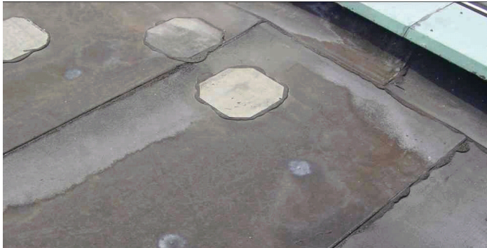
Picture 1: Example of damaged flat roof
