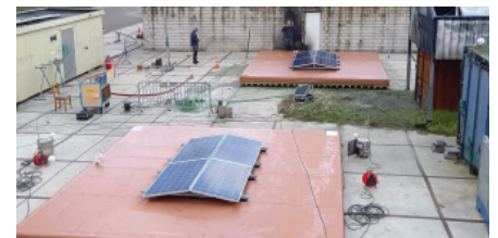
Figure 2: Arrangement of PV system on the roof
